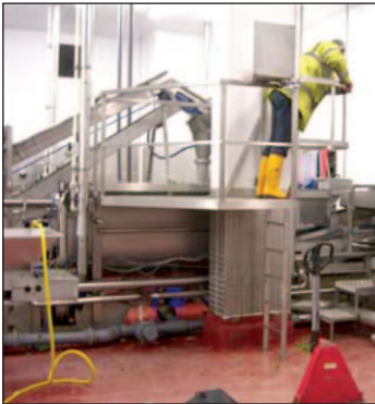
Access gantries and platforms
